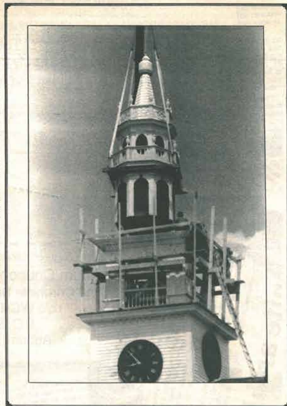
The re-attachment of the repaired steeple to the Jaffrey Meeting House was a welcome and much-photographed sight in Jaffrey.
